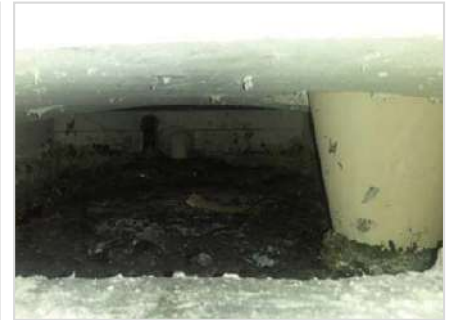
Figure 7: Condition of furnace after 3.5 years
